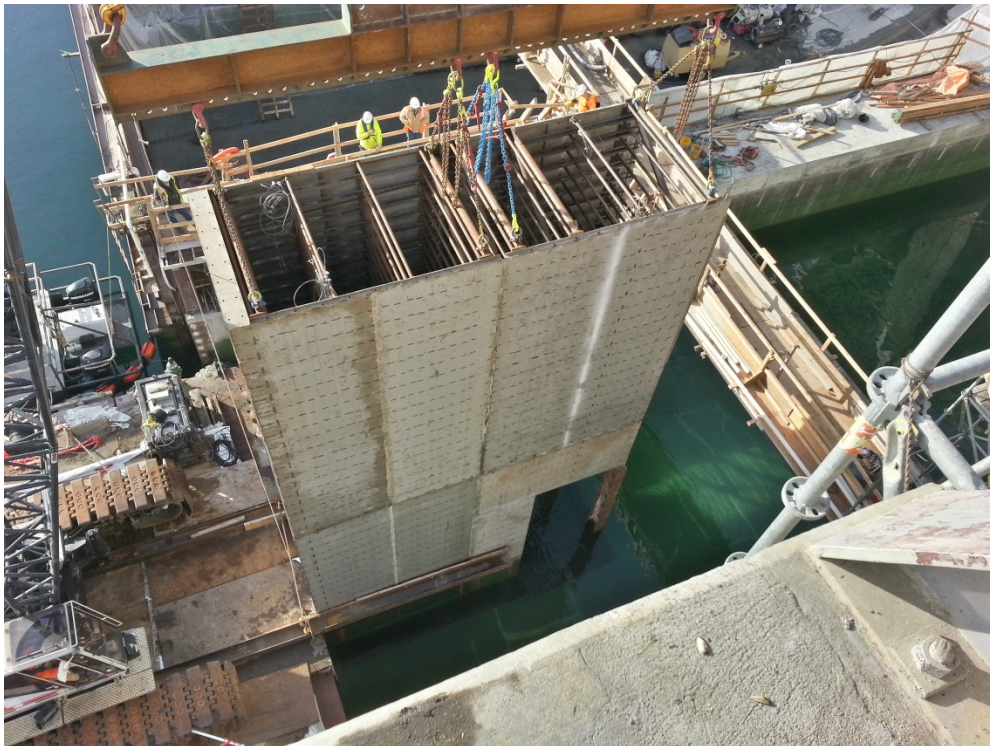
Figure 6 Priest Rapids Fish Bypass. Pier Tail Structure 23 Being Staged in Bay 22, Prior to Setting on Pier 23 Foundation, December 2013.
