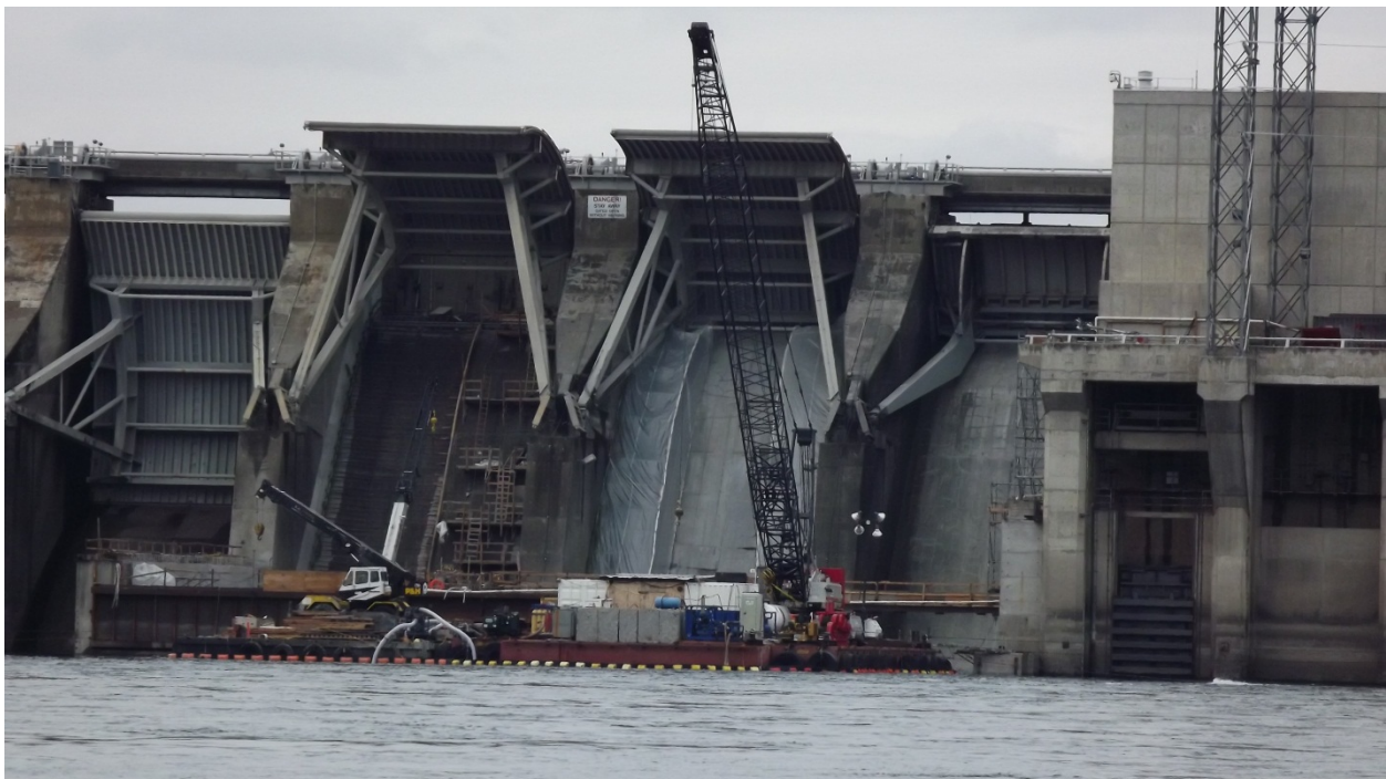
Figure 4 Priest Rapids Fish Bypass Construction Activities. Looking Upstream at Gate(s) and Spillway Improvements, December 2013.
