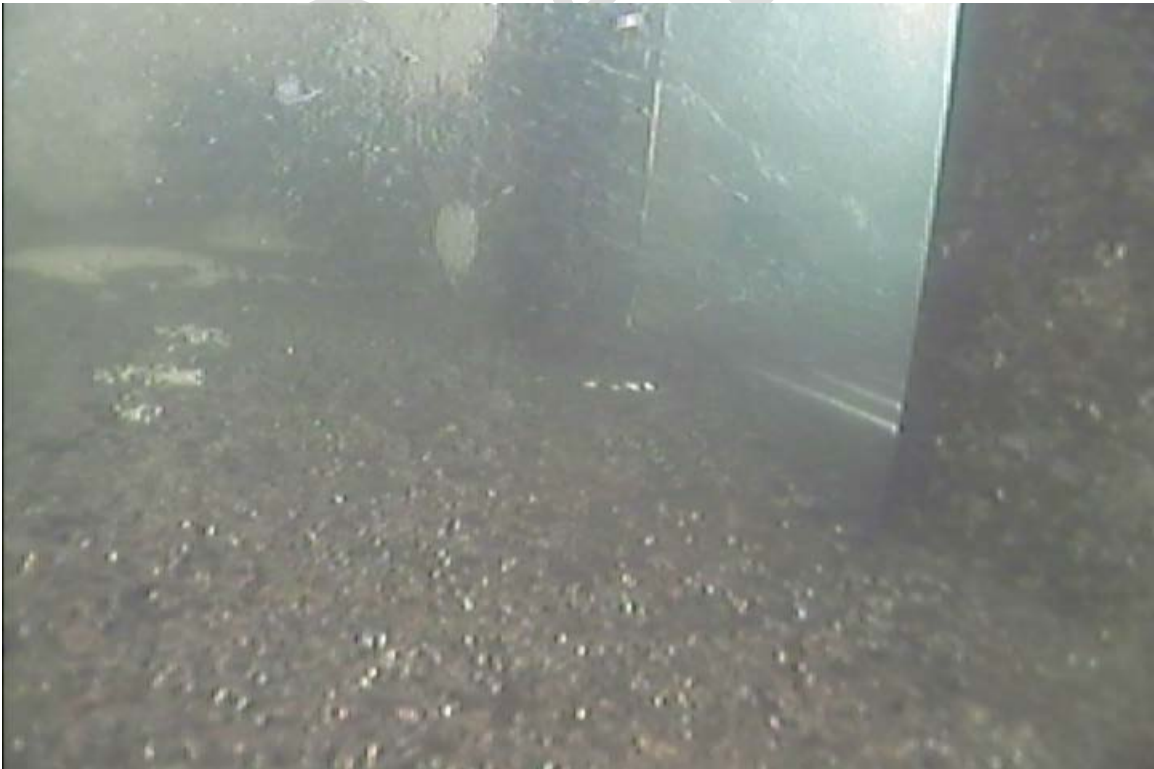
Figure 19 Adjacent to Location F looking downstream at orifice when entrained air was low.
