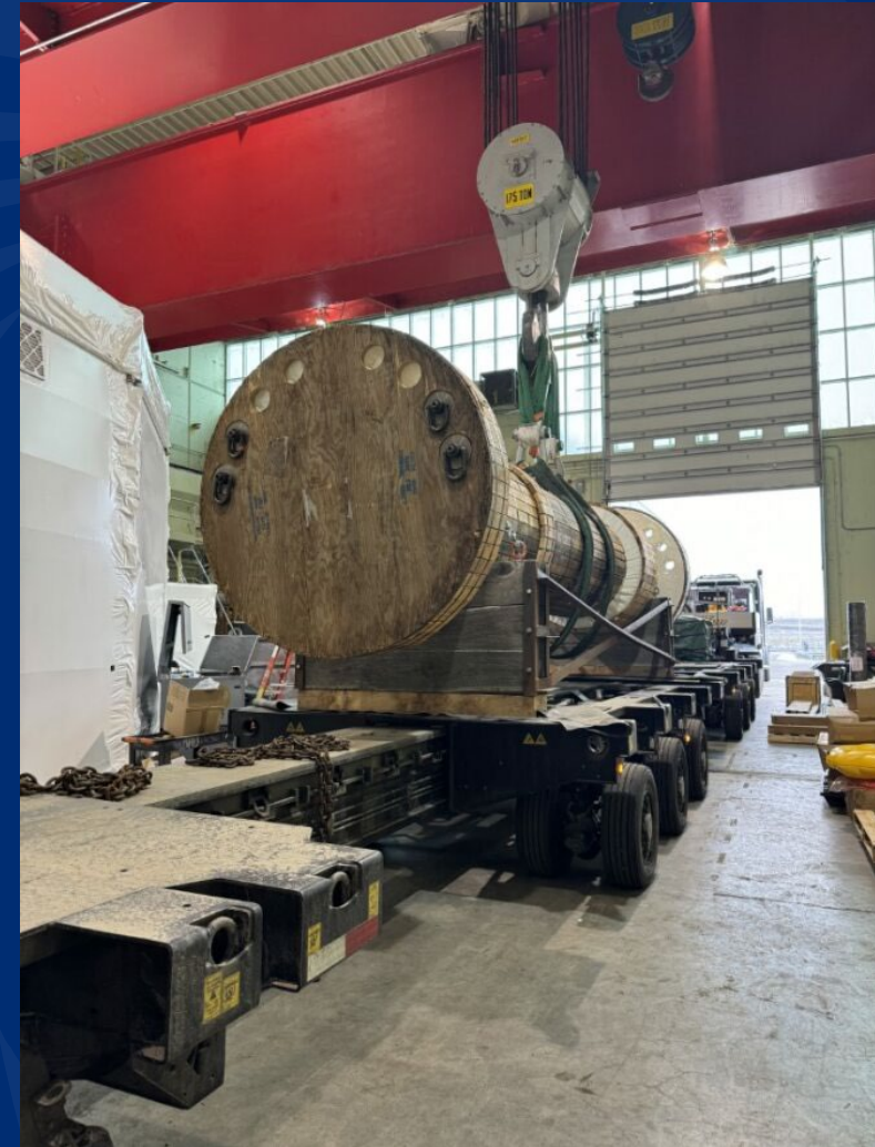
PR Unit Rehab (P1), Turbine is Removed. Picture of shaft being sent out
