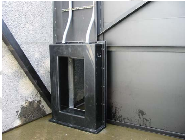
Figure 3 PIT-tag antenna mounted to the upstream side of the VFC box of Weir 7 in the Priest Rapids Dam east-bank adult fishway.
