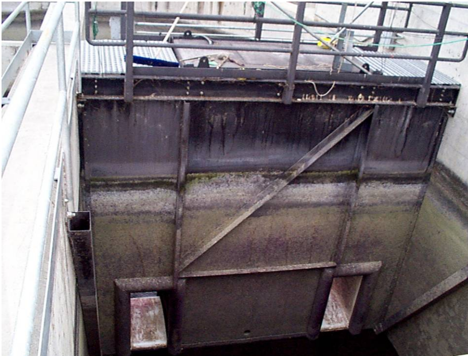
Figure 1 Wanapum in-ladder camera box with fishway dewatered
