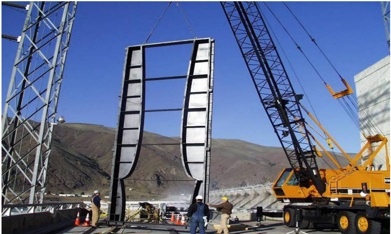
Figure 2 LSE-4 installation at Priest Rapids Dam, Columbia River mile 397.1, Washington, USA, winter 1998-1999.
